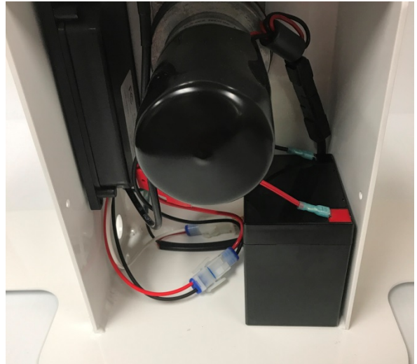
Properly installed battery
